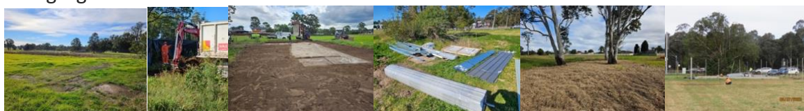
From Left: The worksite selected for installation of a small secure storage shed; Work to decontaminate the site of asbestos; the worksite after decontamination work was completed; the original shed material – before the theft in August; Removal of Alligator Weed along Bells Creek has progressed; Installation of security fencing to protect the shed has commenced in July 2025 (Images: R Howitt)
